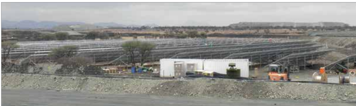
Fig. 3.18: Solar energy plant at Thaba Mine (photo: DERA 2012).
