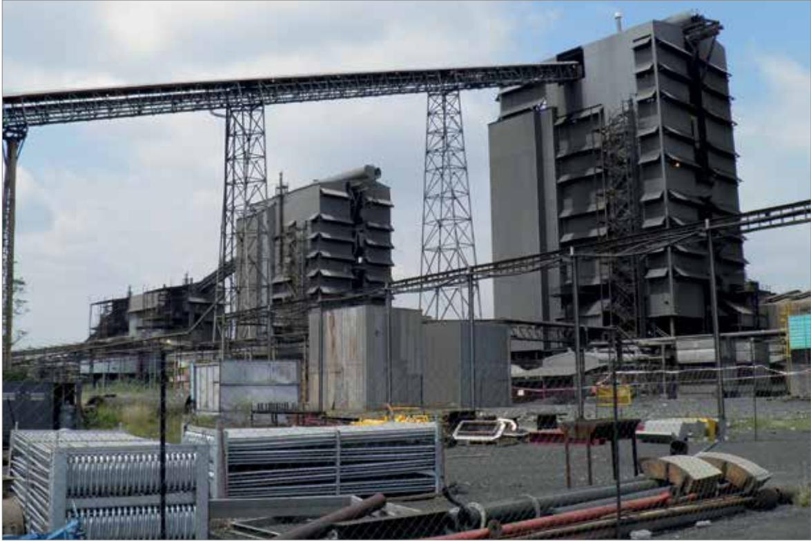
Fig. 3.20: The four intermittently tapped electric furnaces at Heric Ferrochrome (photo: DERA 2013).
